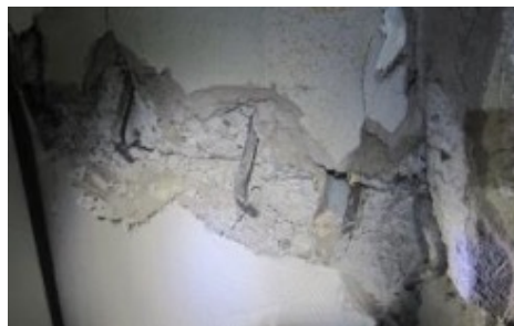
Figure 4 Single crack opening of wall with low long. reinforcement ratio (NZSEE et al., n.d.-a)
