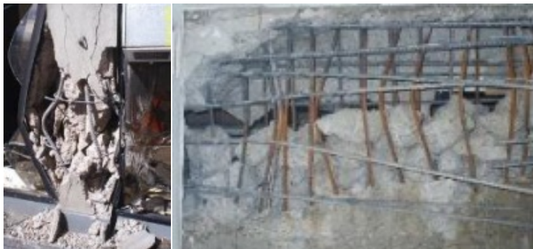
Figure 2 Failure due to inadequate transverse reinforcement and confinement (NZSEE et al., n.d.-a)
