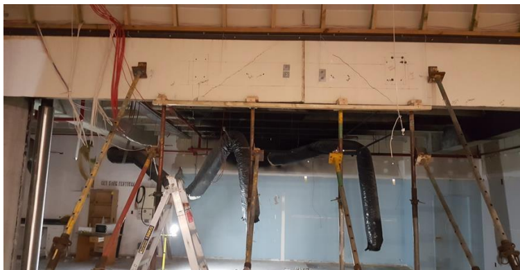
Figure 1: Compromised basement construction
